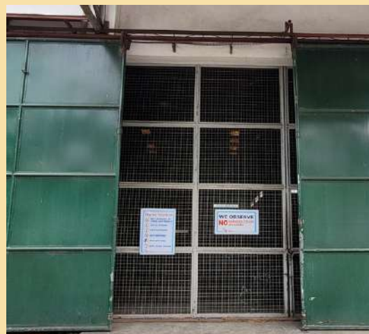
Image 21. Warehouse opening or doorway with mesh screens (Photo taken at NFA East District Warehouse)
