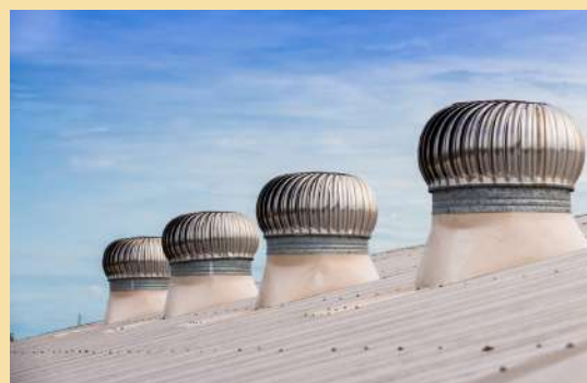
Image 12. Warehouse rotary ventilation (Karnnapus, n.d.)
