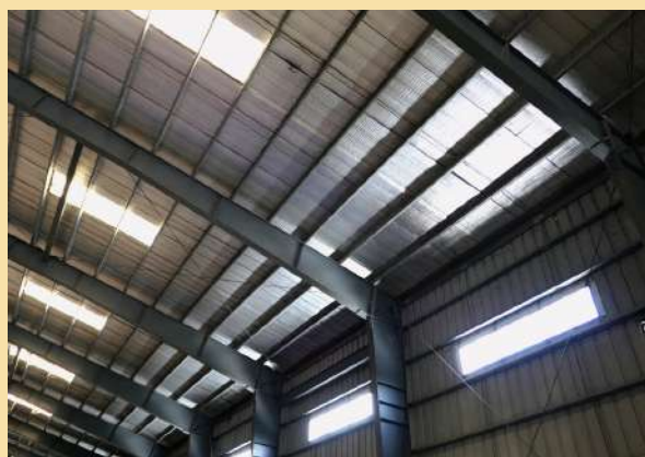
Image 25. Warehouse roof; no opening between the wall and the roof (Photo taken at NFA ACA warehouse)
