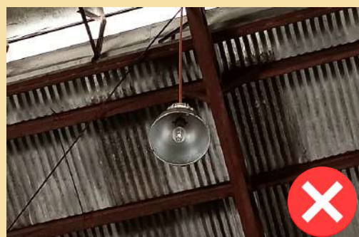
Image 24. Lighting fixtures without enclosure
