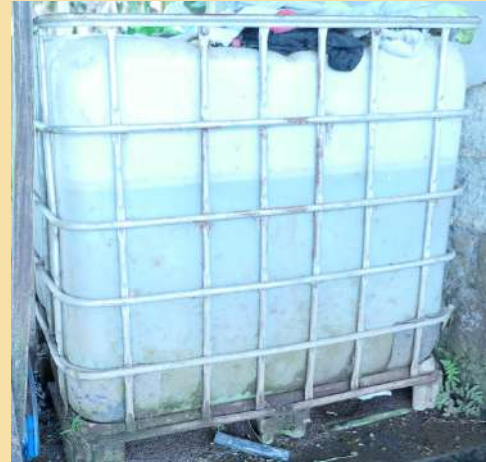
Image 44. Additional water tank in case of power interruption
