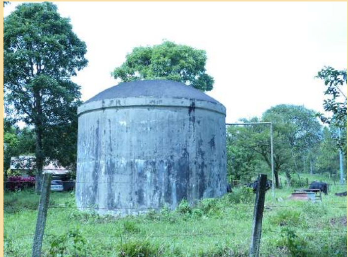
Image 12b. Water tank
